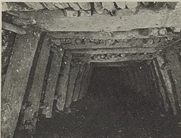
Fig. 1—Gangway Section, Showing Forepoling in Crushed Ground. Timbers Have Been Standing Sixteen Months.
