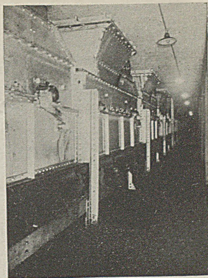
Lighting a Conveyor Gallery
