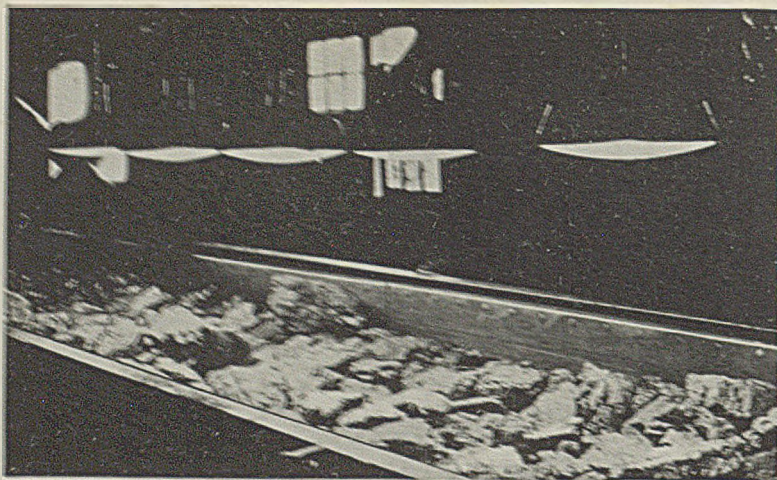
Electrical Daylight Facilitates Picking Where Dust-Tight Cover Glasses Are Easily Accessible for Cleaning
