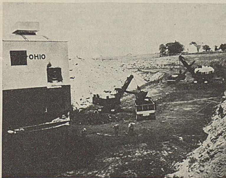
Fig. 1—View in the Pit at Mark Twain, Showing Cleaning Method and Loading Shovels at Work in the Mulky Seam.
