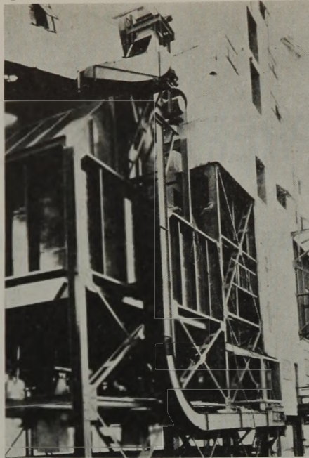
Redler Installation at New Orient.
