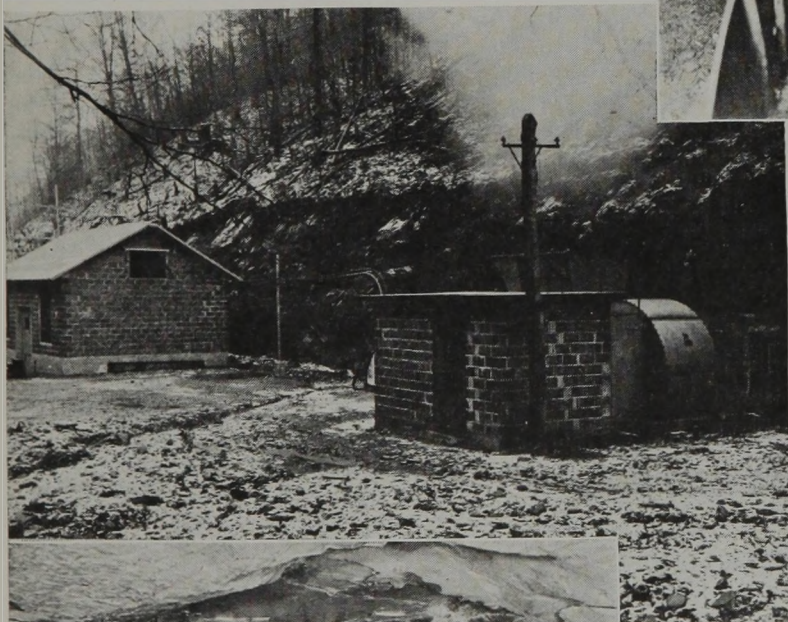
Substation and Fan, Representing the First Move in Raising Loading Efficiency in No. 9.
