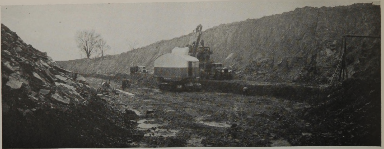
Loading Shovel Cleaning Up Along the Coal Berm on Which the Trailer Units at the New Delta Strip Mine Operate.
