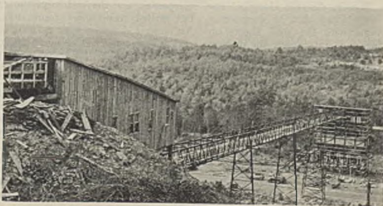
Fig. 1—Plant of Gunton Coal Co. during construction. Crusher house on left; breaker on right
