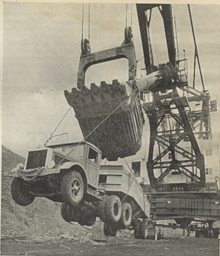
Close-up of the 30-cu.yd. Bobolink stripping unit toying with one of the 25-ton trailer units
