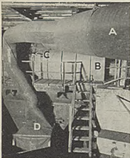
"A" is the branch duct to the dump; "B," the dump inclosure; "C," one end of the operator's window; and "D," the inclosure and curtain at the lower end of the feeder
