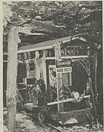
Operating view of the semi-automatic control truck showing the steel-canopy roof protection
