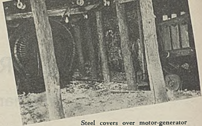
Steel covers over motor-generator and control truck units obviate any necessity for building a room for portable substation operation. This is an operating illustration of a 300-kw. unit in New Orient mine.
