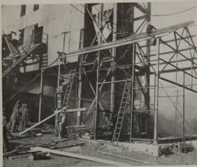
Large Dimensions of the Skip Shaft Radiator Building Shown in This Construction View.
