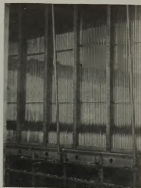
Radiator Sections Viewed From Inside of the Building. Bright Sunlight Appears Coming Through the Air Spaces Between Tubes.
