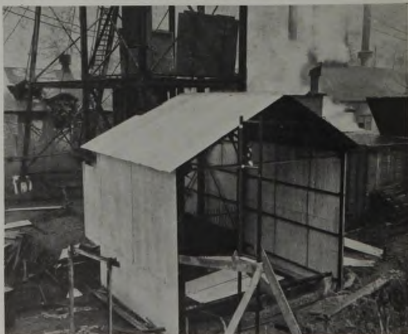
Airlock Doors of the Auxiliary Shaft Appear at the Top of This Construction View.
