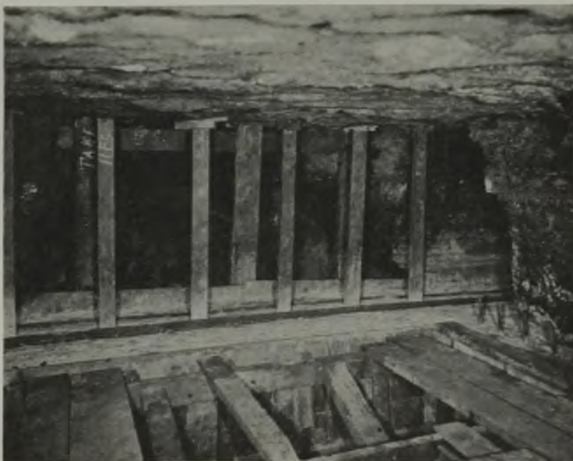
High-Pressure Seal at End of First Stage of Construction, Showing Bottom Portion in Place and Vertical Reinforcements in Position
