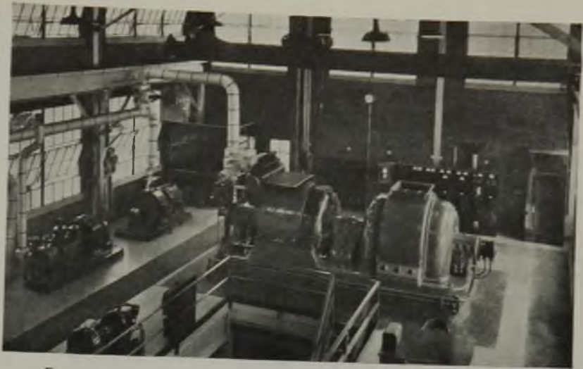
Present Loads Are Carried by This 3,000-Kw. Turbo-Generator.
