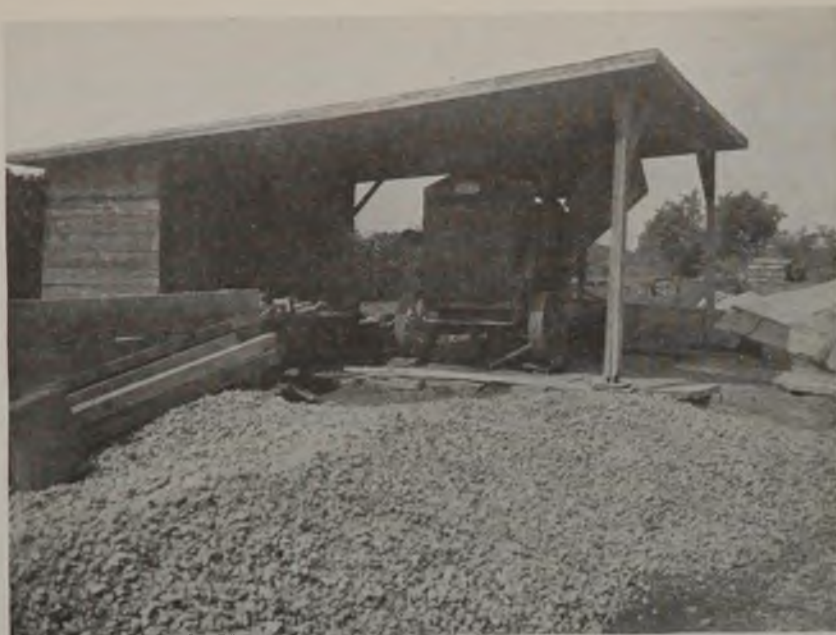
Concrete Mixing Plant on the Surface. Mixer is Located Across Supply Track From the Cement Storage Shed, With Gravel and Sand Yards to the Left and Right of the Mixer, Respectively
