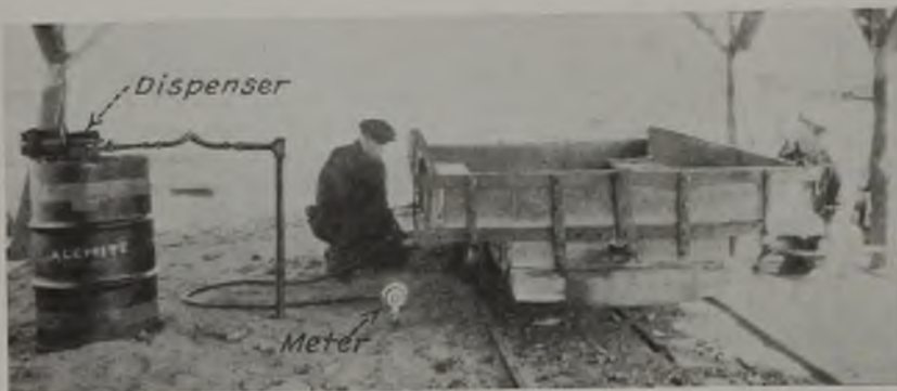
Car-greasing station and equipment at Mary Helen mine. Pipe connections serving the two hoses through meters are buried under the tracks
