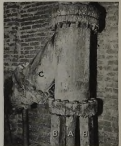
"A" is the electrical conduit; "B" are construction supports left under the discharge column; and "C" is the discharge pipe from the pump
