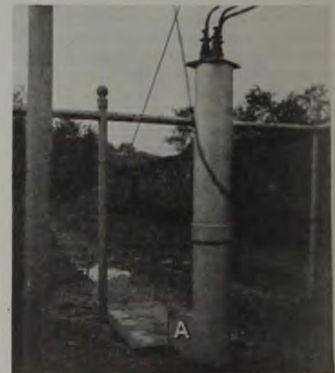
"A" is the water-discharge opening below the pothead
