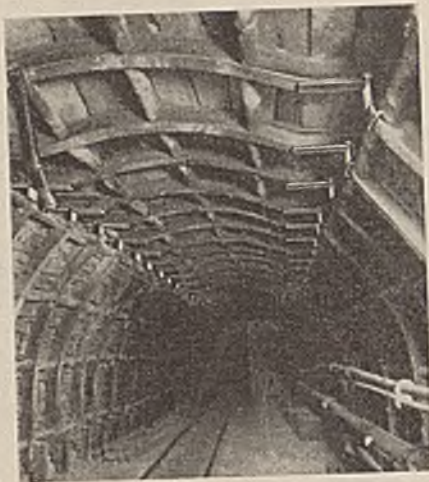
Fig. 2—With Yielding Angle Joints, Peg Legs, and Curved Members, Lining Gives Without Collapse
