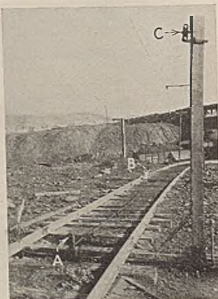
Fig. 1—High End of Switch Control
