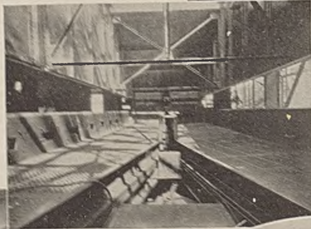
Construction View of Pri- mary Table Before Wooden Decks and Tanning Cloth Were Applied. Note Refuse Discharge Openings Along the Sides
