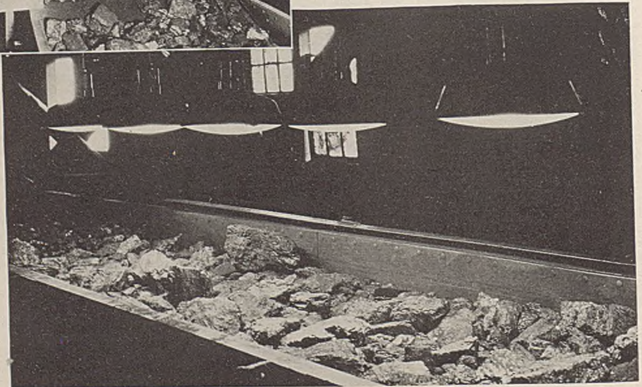
Fig. 2—Electrical Daylight at Work Over the Coal Picking Table. Note Ease of Vision and Also Ready Access of Dust-Tight Cover Glasses for Cleaning
