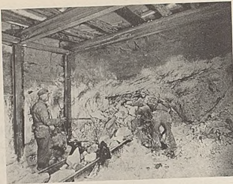
Fig. 2—Handling Sandrock by Duckbill in Sidetrack at Winton; Note 17-Ft. Steel Sets
