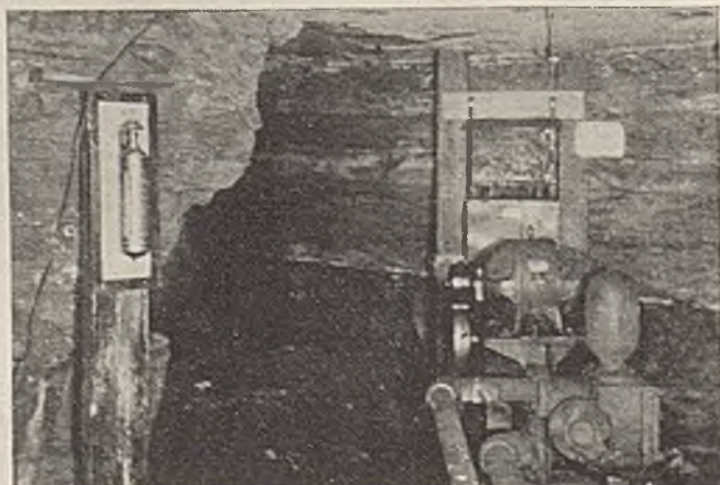
The Extinguisher Is More Prominent Than the Motor
