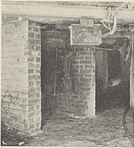
Reclosing Circuit Breaker Protected by Brick Vault
