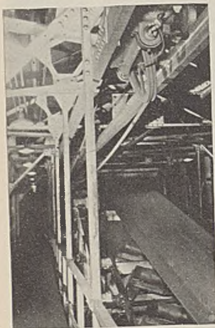
No Arcing Involved in Feeding This Traveling Tripper
