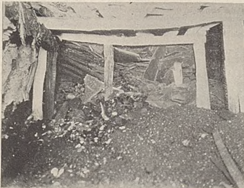
Systematic Mining Causes the Roof to Fracture and Fall on the Line of Solid Coal
