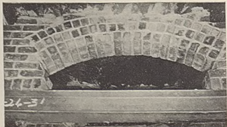
Fig. 3—Under Moderately High Roof an Abbreviated Arch Is All That Is Required
