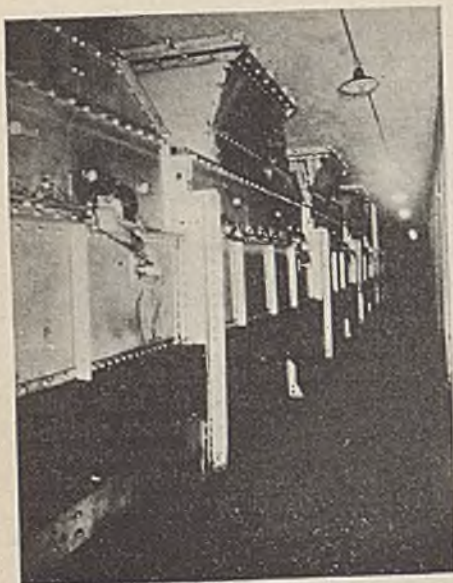
Fig. 4—Where Coal From Bin is Fed to Lower Strand. Gallery Looks Level but Is on a Steep Pitch
