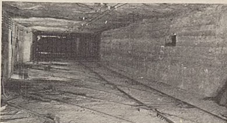
This Barn Accommodates 24 Battery Locomotives. It Is in the No. 14 Mine, Consolidated Coal Co. of St. Louis
