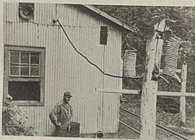
Resistance Coils in Feeder to Trolley Wire
