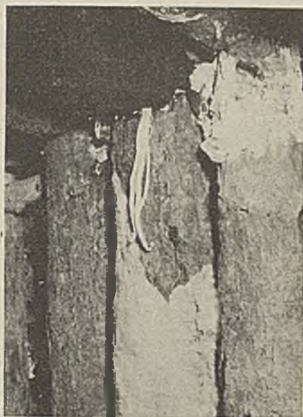
Solid Treated Timber and Decaying Untreated Posts
