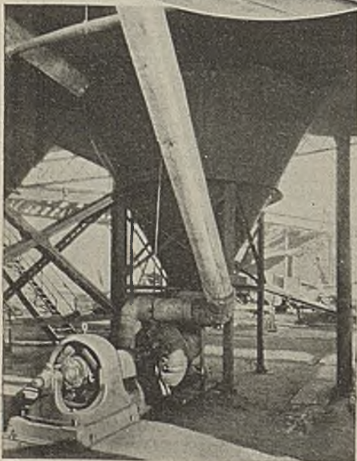
Fig. 5—Storage Tank and Circulation Pump
