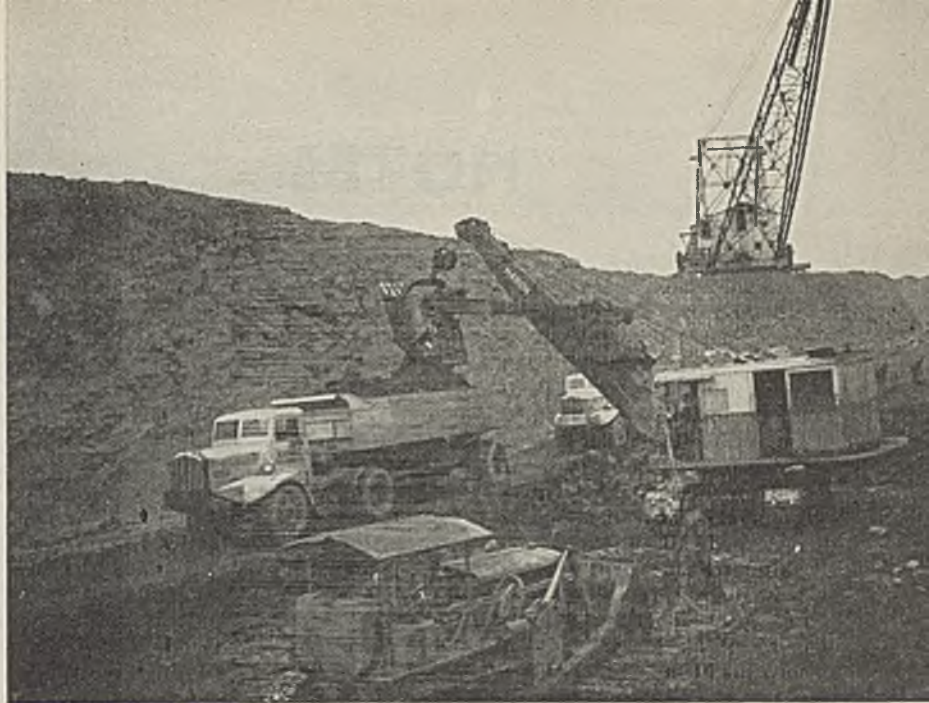
Loading in the pit with the new diesel-electric shovel and tractor-trailer haulage units
