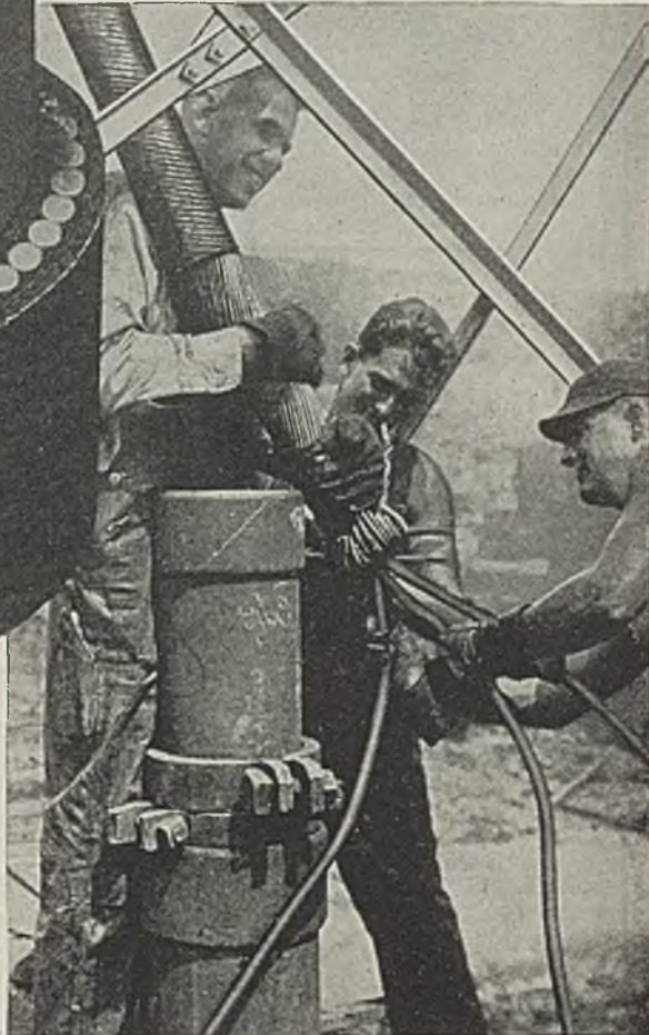
Hazard Steel Armored Borehole Power Cable being lowered through an 8" borehole and supported by steel tower.
