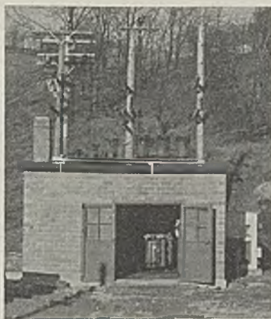
Fig. 1—Rectifier substation, Crescent No. 2 mine
