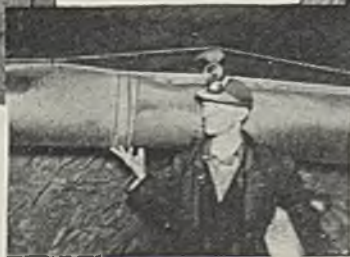
(Below) The regular type flexible "Ventube" carries fresh air to remote headings, forcing dust back away from the working face.
