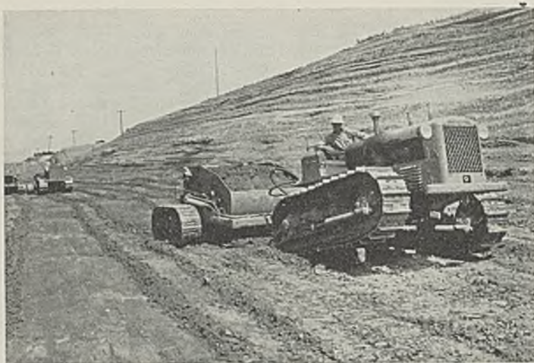
Tractor-powered scrapers working in the railroad cut made to reach the site of the preparation plant
