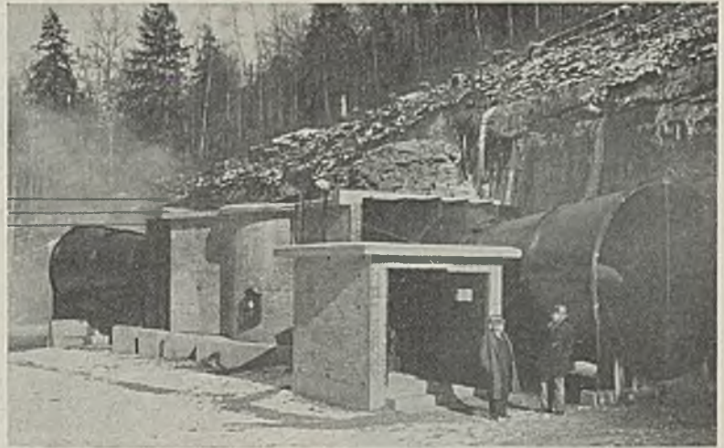
Two propeller fans operate in parallel at the top of the new air shaft
