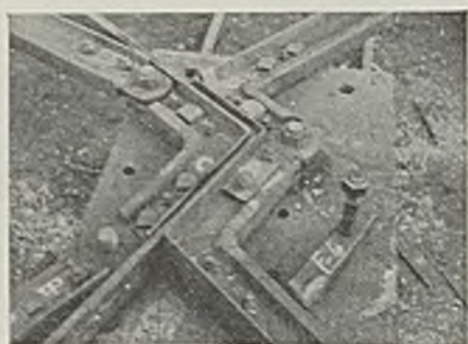
Fig. 16—Showing Bend No. 2 completed and Rail Lock F-6 against Rail A-1 ready for Bend No. 3, which is followed by Bend No. 1
