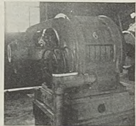
Neatness assured in wiring this wound-rotor motor.
