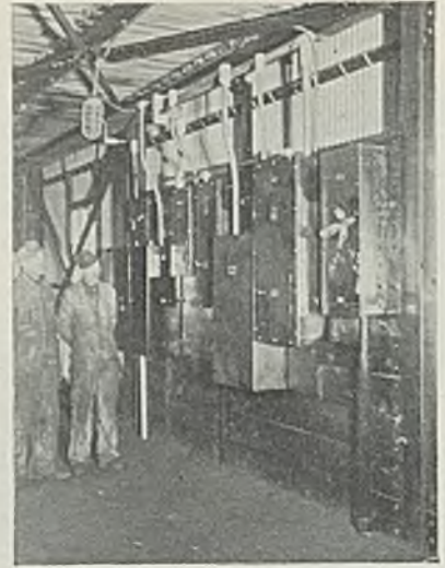
Headhouse electrical controls are grouped on a floor beneath the track. James Tolbert, construction electrician (left), and C. H. Price, chief electrician (right), view the finished job.
