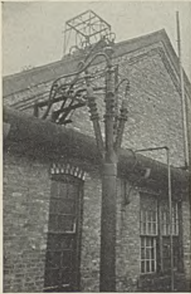
Top of borehole near the shaft at No. 2 mine. This 8-in. hole carries a 2,300-volt a.c. cable; two 1,000,000-circ.mil d.c. positive circuits, three 500,000-circ.mil return lines (all held by one clamp), and telephone and light circuits.
