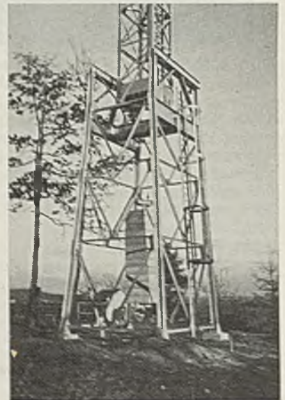
Base of the tail tower, which was erected bottom section first, top section second, next to top section third, and so on.
