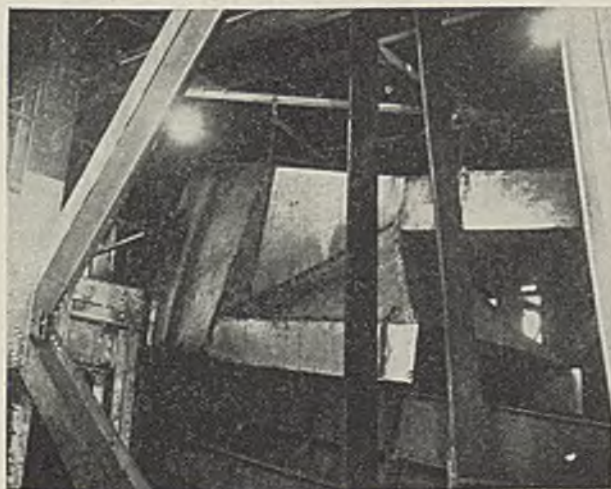
Part of the Isabella dust-collecting system—hood over the scalping screen with duct to exhaust fan.
