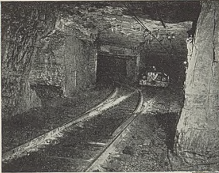
60-lb. main-line turnout, using low-type parallel-throw switchstand and cast-manganese-steel shrouded frog. This turnout had not been cleaned in six months. Ties are treated.
