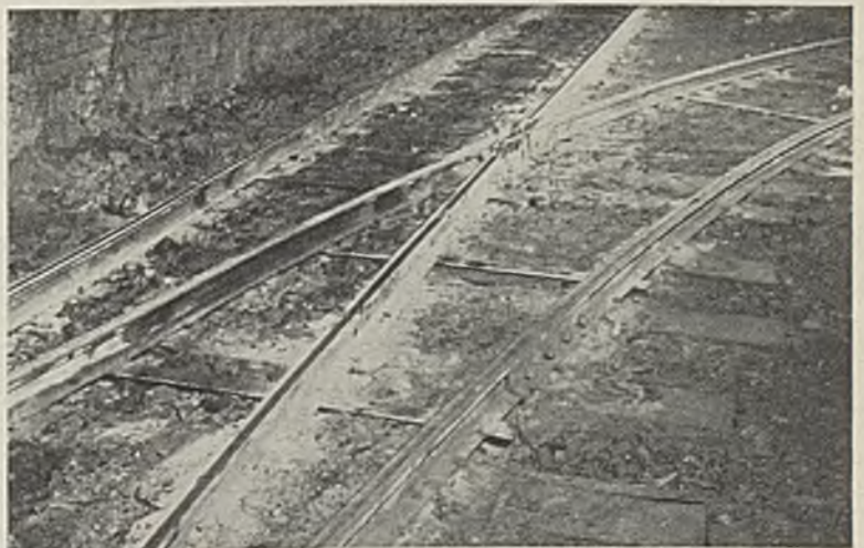
Cross rails are used as bonds on main-line track, as indicated in this view of a 60-lb. turnout.
