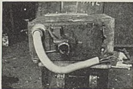
Fig. 5—Airplane tubing originally employed for a gas-tight connection between controller and machine, which was disapproved by the State electrical inspector
