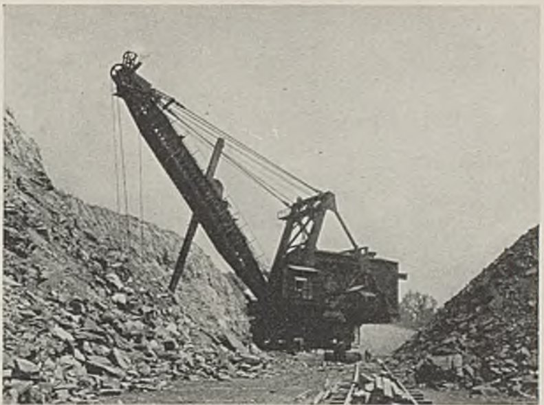
Stripping at the Ayrshire pit. The 15½-cu.yd. dipper on this electric shovel replaced a 12-yd. unit. As holes are "double-decked," 8 to 10 ft. of shot material is left at the top of the bank, as detailed in the accompanying article.
