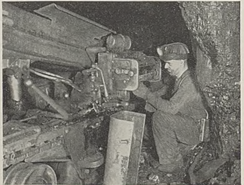
At Miami No. 10, the chief electrician "grabs" this chance during lunch hour to inspect the controller of the loader.
