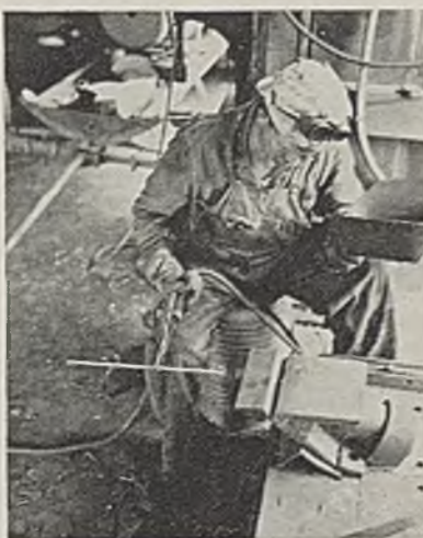
A cast-manganese end, or cutting edge, has been "tacked" in place ready to weld at Minnehaha. The point is held in a special clamp on the bench so that the weld can be peened. Welding the new cutting edge and building up the face will complete the pointing job.
