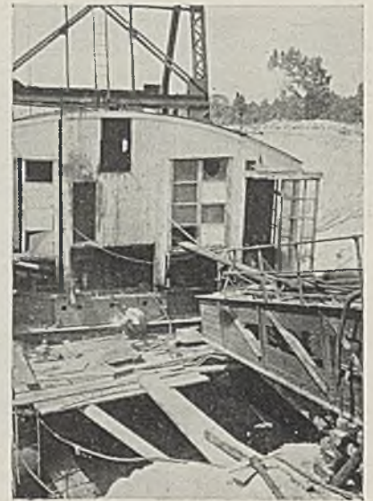
Arc welding a crack in the front girder of the revolving frame on the Clinton stripper.
