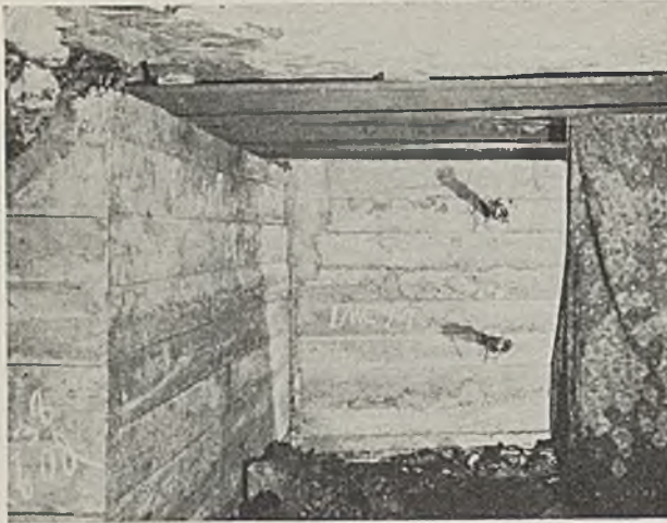
Primary gas seal in Kings Station mine. A line brattice at the right causes ventilating air to sweep the seal. The top is protected by rails set on wing walls.
