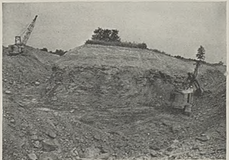
Showing the special stripping shovel digging up the hard material at Star Hill No. 1, which the dragline later will pull back off the coal and spoil.
