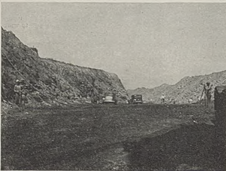
For more efficient shooting, overburden holes at Enos are spotted with a transit, and yardage and charge per hole are figured by an engineer.
