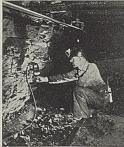
Chief Electrician James Tweedy demonstrates checking bonds by measuring current in the negative return wire.
