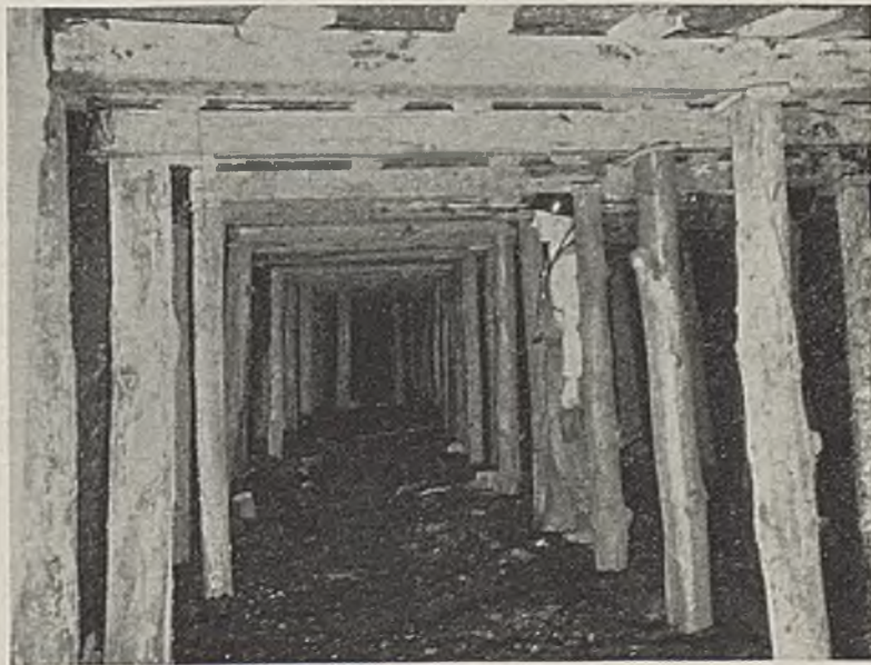
New aircourse timbering system at Talleydale, showing treated wooden bars with three treated legs which replaced steel-rail bars on two untreated legs.
