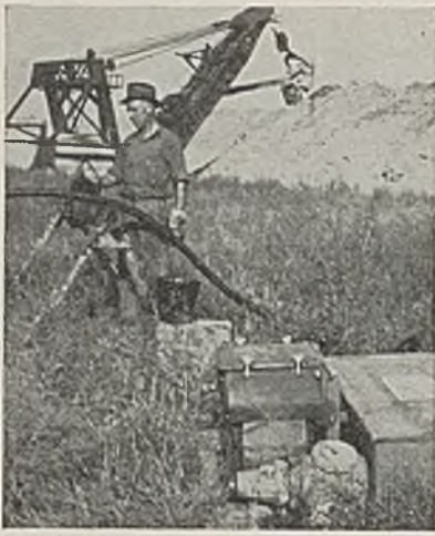
Painting the trenchlay field cables at Linton Supreme No. 23 to reduce abrasion of the jute covering.
