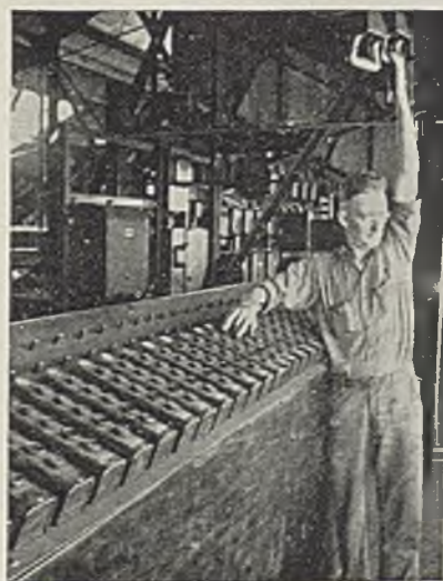
Twenty-seven interlocked pushbutton stations control the new Minnehaha plant.
