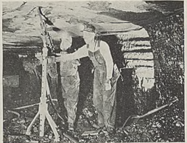
Cutting hitches for seals at Kings Station. This air-driven paving breaker is used for cutting top and bottom. The rib hitch (right) was outline-drilled and shot.
