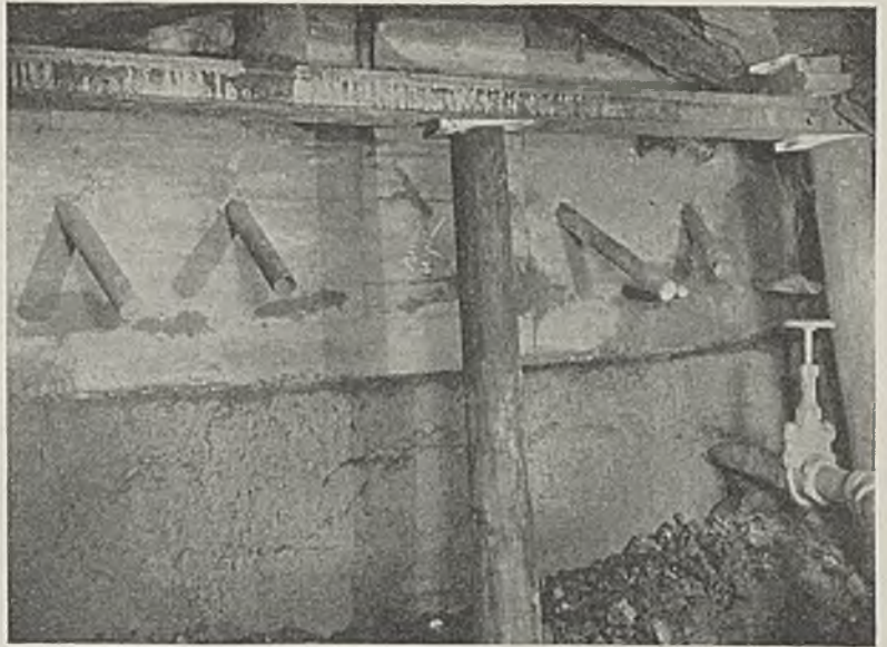
Several grouting pipes in the top half and a water pipe in the bottom section can be seen in this 6-ft. bulkhead just completed in Saxton mine. The panel is filling with water and the pressure probably will reach 60 lb.
