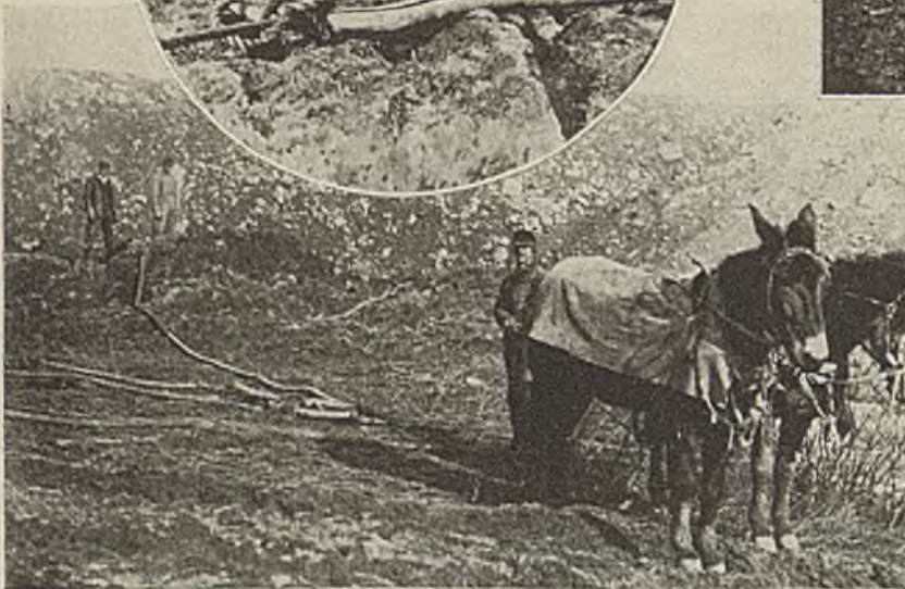
In Circle—Hitching for Dragging 4,000-Volt Cable; Here It Happens to Be Attached Next to a Bronze Sleeve Covering a Splice in the Cable
