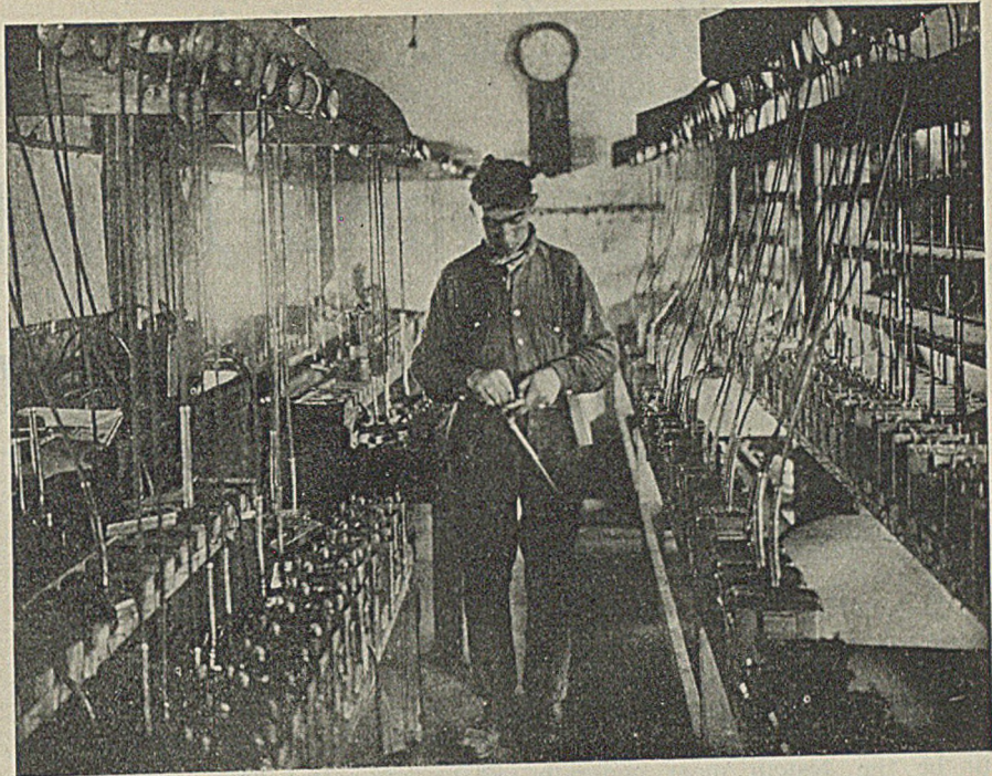
Battery Charging Room for Cap Lamps
