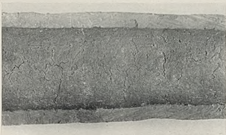
FIG. 19.—Lead Pipe Failed in Service while Carrying 70% Sulphuric Acid at 140° C.; Vibration due to Adjacent Motor.
