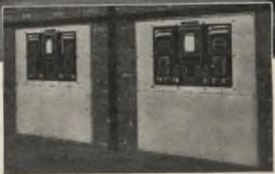
The Control Boards.
