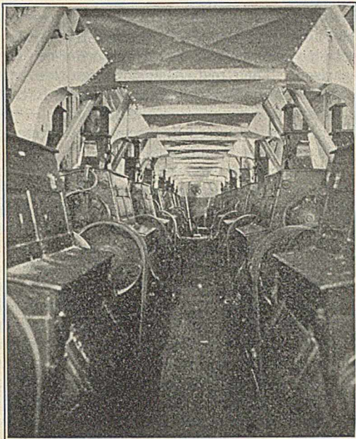
Air Conditioners in Flour Mill of J. Allen Smith Company
