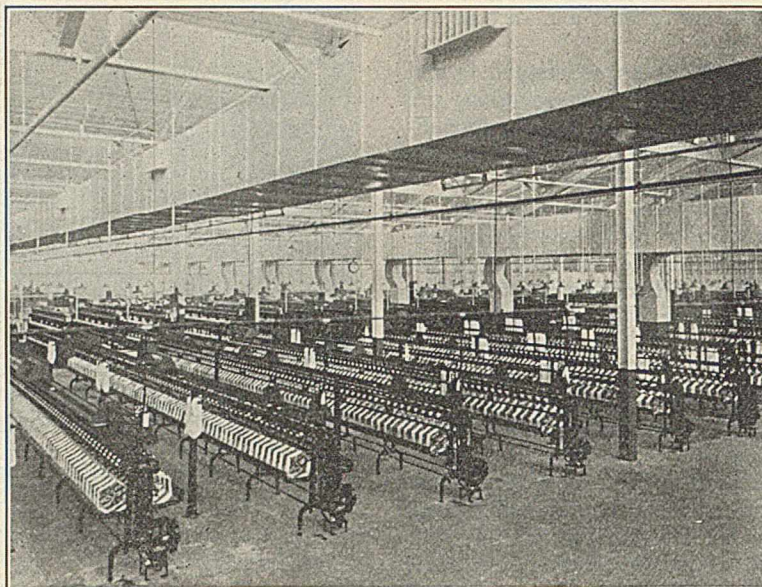
Winding Room in Rayon Plant of the American Bemberg Corporation Conditioned air is distributed throughout the department through diffuser outlets shown in the metal duct near the ceiling.
