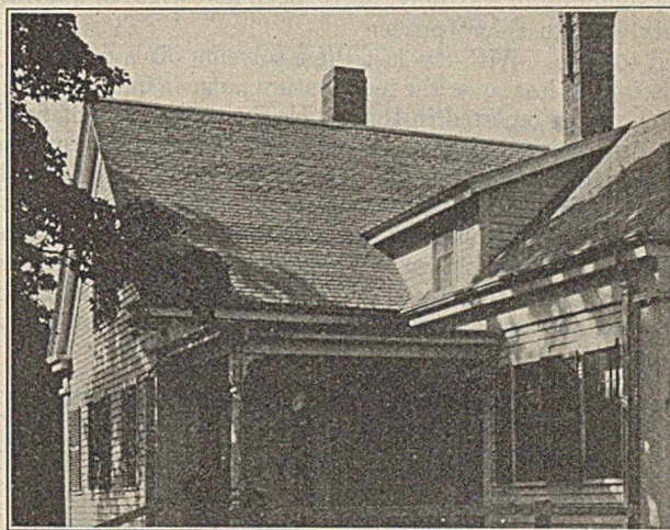
Figure 2—Roof of Asphalt Shingles on Which Curling Has Occurred
