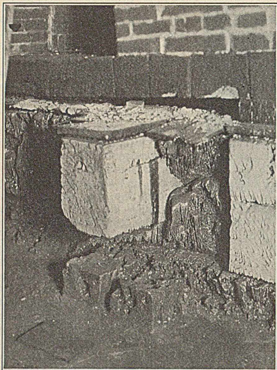
Figure 5—Comparison of Corhart Blocks with Ordinary High-Grade Refractory in Glass-Tank Service
