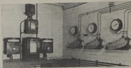
FIG. 15.—ANNEALING OVEN PYROMETER CONTROL ROOM.
